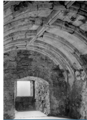
The ribbed, barrel-vaulted ceiling in the third floor chamber of the tower, probably added c1600 Crown copyright: RCAHMS
